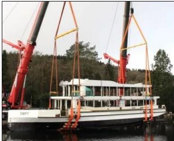
The launch of MV Swift into Lake Windermere by two 500 tonne mobile cranes
