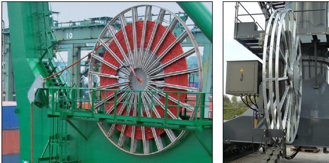
Examples of power cable reel systems installed on dockside cranes
