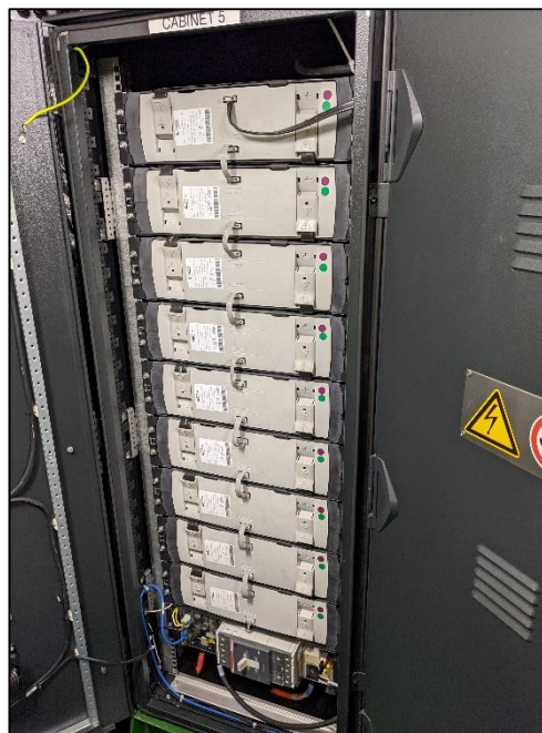
One battery bank module of an electric ferry
