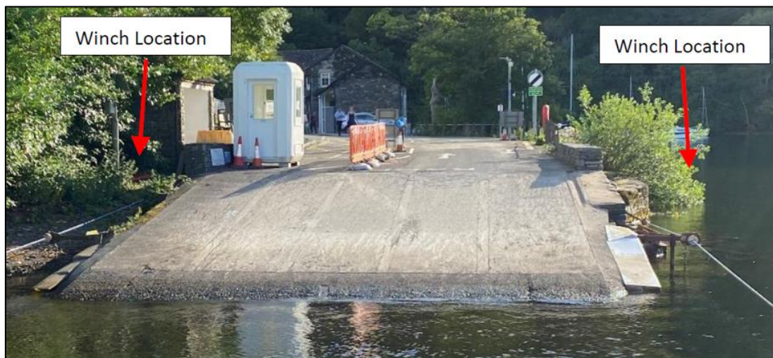
The Ferry House (west) slipway showing indicatively the location of the winches
