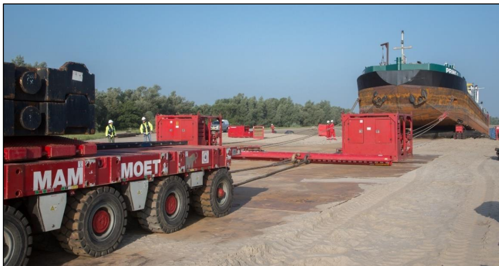
Example of hauling a vessel up a slipway (courtesy of Mammoet UK)
